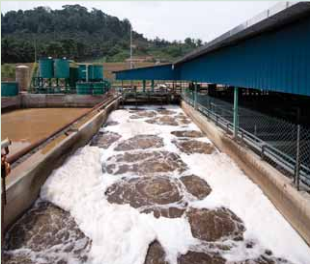
KKI treating wastewater at the ETP
