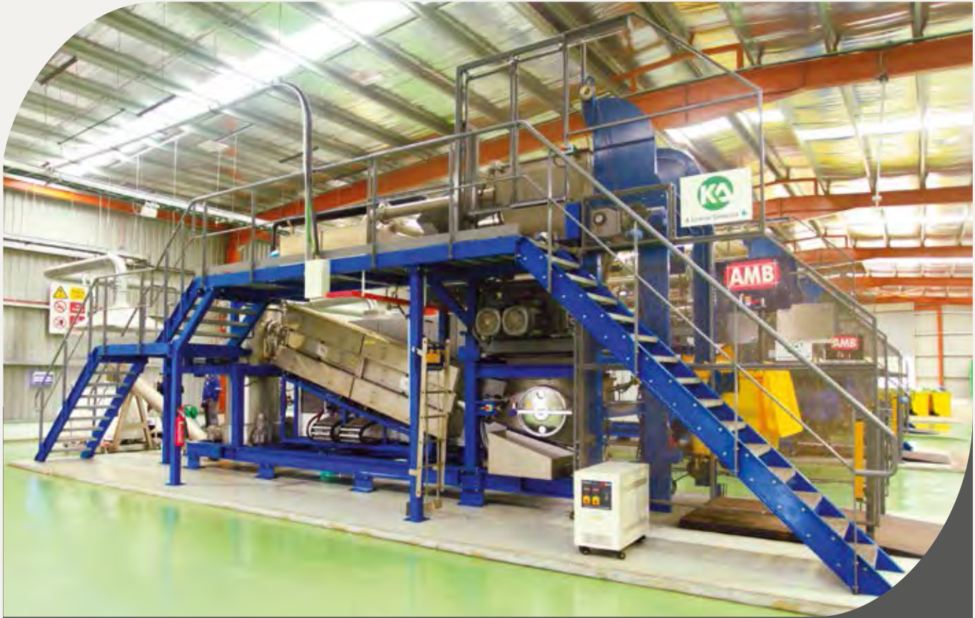
Malaysia's 1 st non-incineration CWTC
